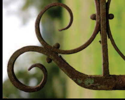
Light rusting of ironwork
