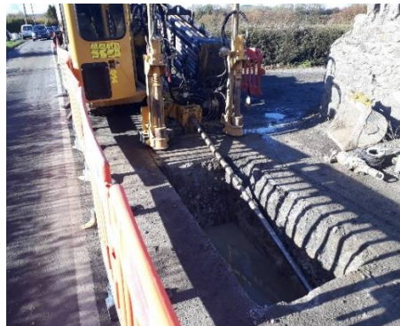
Installation of a new watermain in Freshford (work being carried out under the Water Network Programme )
