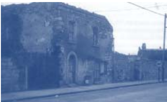
Before ..... Derelict Sites at Barrack Street, Goresbridge
