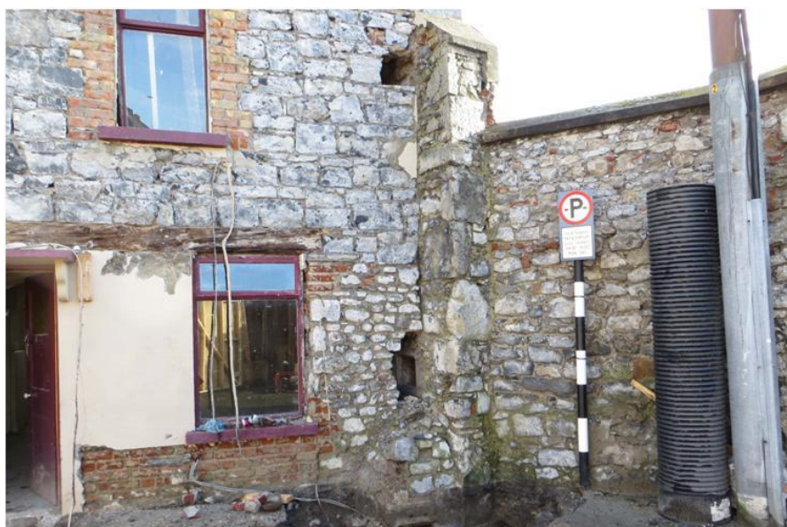
Plate 3: Buttress at front of 22 Vicar Street
