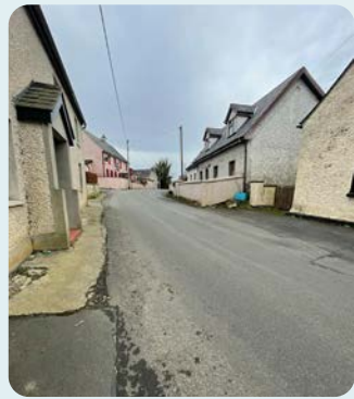
Figure 3.37: Poor existing Footpath Arrangement at Kilmacow Lower
