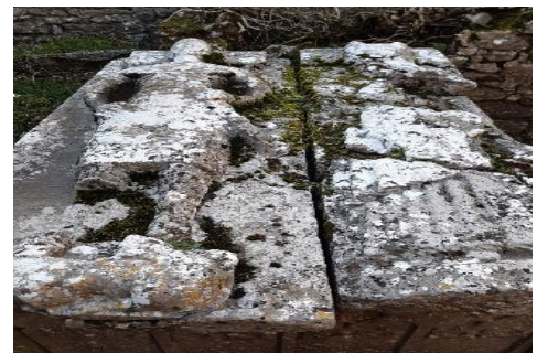
The MacGiolla Phadraig Tomb, Grangerfertagh will be addressed in the Conservation Plan
